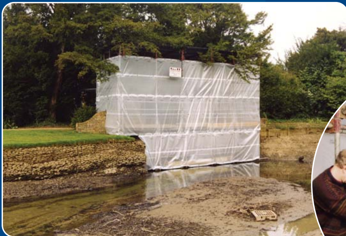
Scaffolding and weather-proofing were erected over the site to comply with health and safety regulations.
