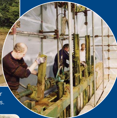
The removal of the top section of the sluice gates including gear components and downright supports.
