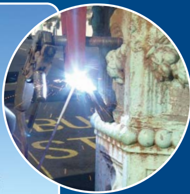
A specially designed reaming cradle was secured around each lamp base to aid accurate positioning of the reaming tool.
