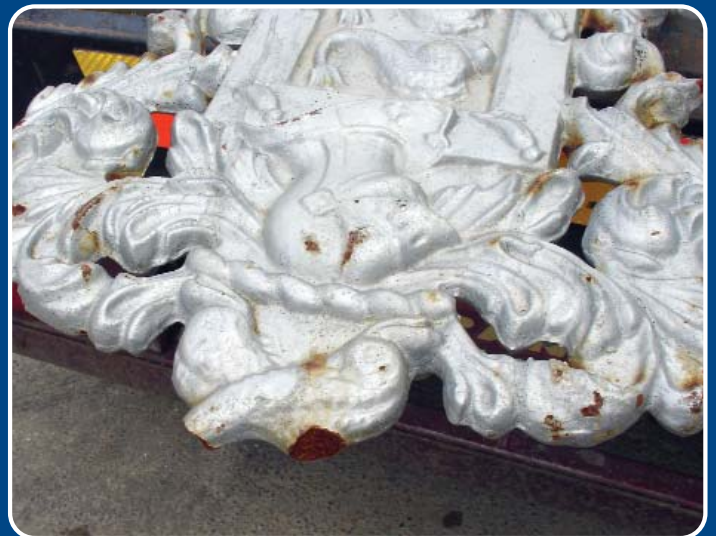
Each of the castings was assessed for damage and subsequently repaired at our workshops.
