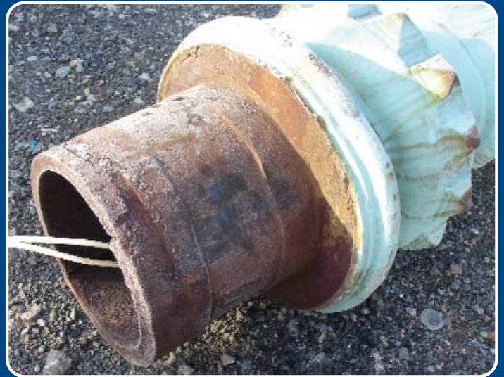
Spigots that locate the columns into the base's were worn, allowing the the lamps to rock dangerously.
